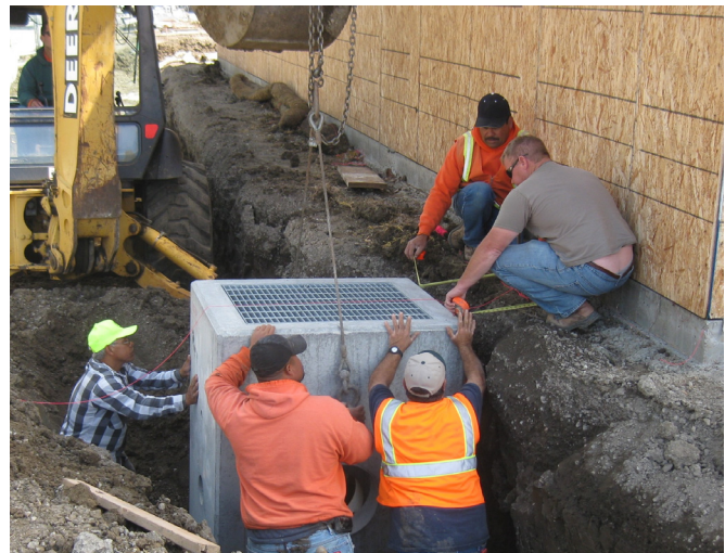
Carefully setting in place the overflow structure for a bioretention facility in Pittsburg.
