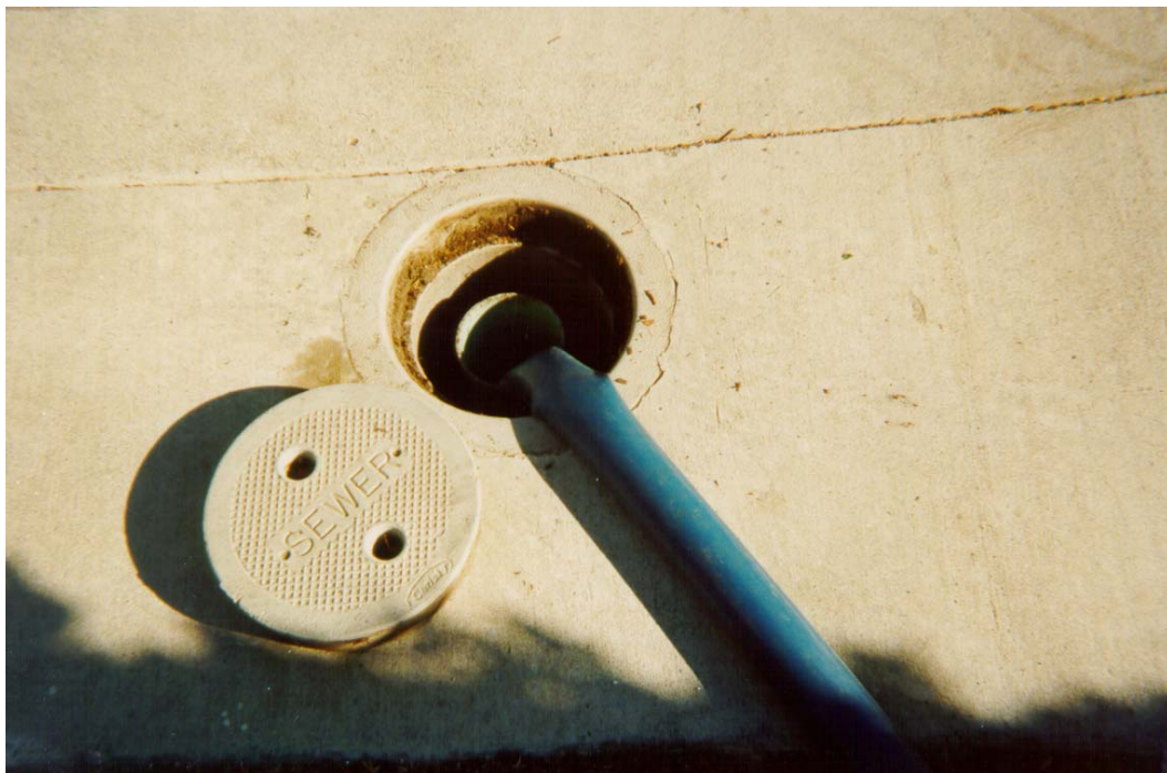
Discharge to the Sanitary sewer at PRIV-07
