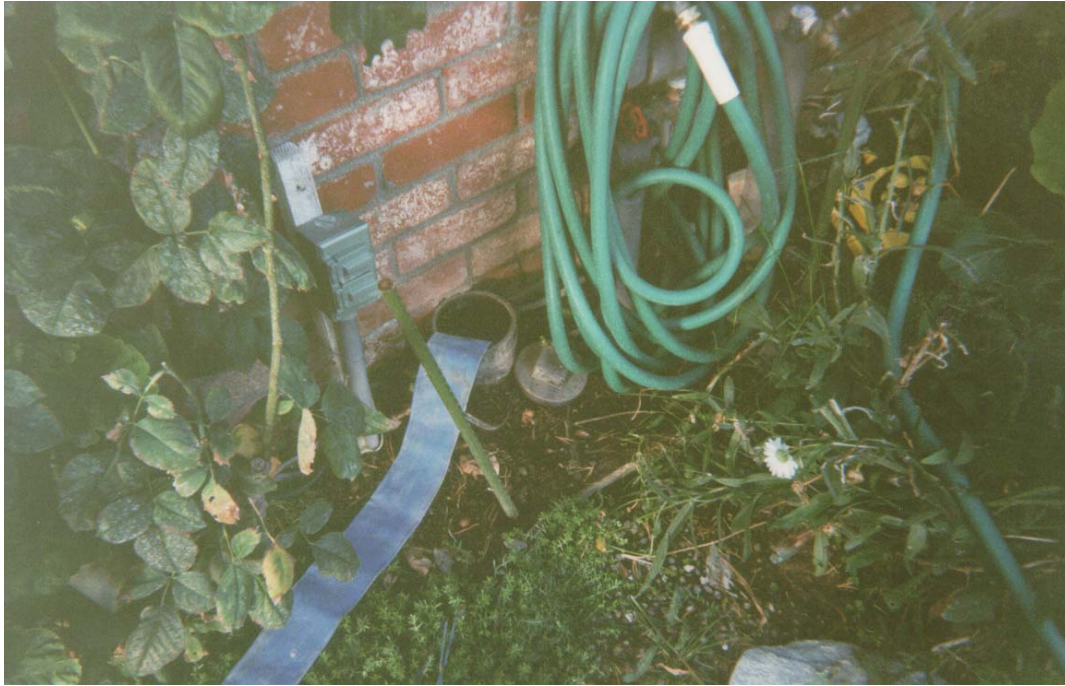
Discharge to Sewer Cleanout Line at PRIV-02
