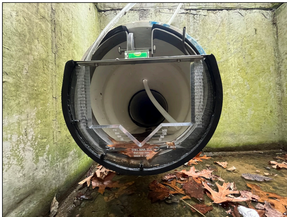
Figure 6. Ohlone Greenway Effluent Weir and Sample Intake Tubing
